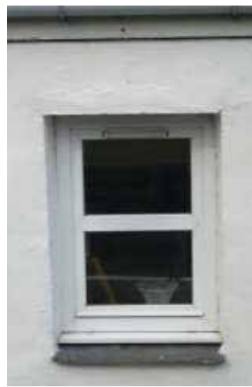
Window not in keeping with the character of the area
